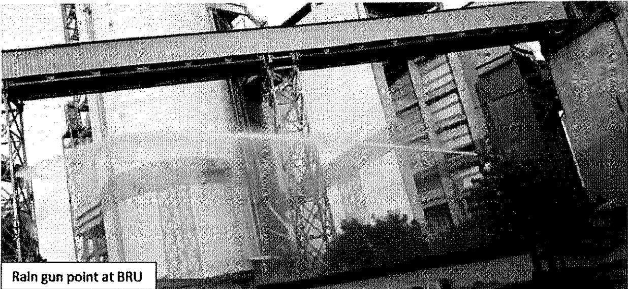
Rain gun point near Fly Ash unloading point
